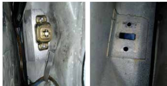
L/H 1987 door with new DOOR ARRESTOR installed
